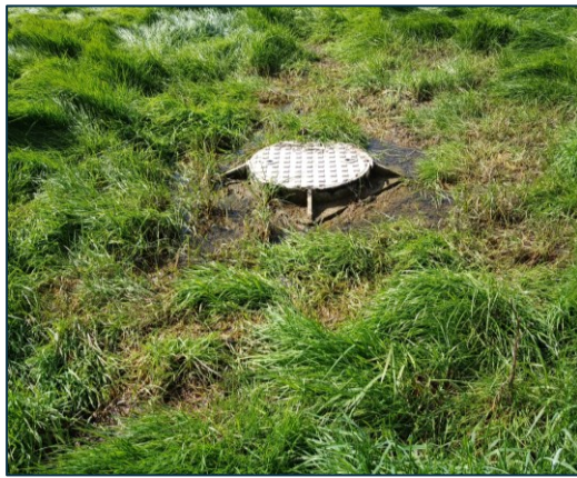
Drain in pasture field, appears to have overspilled.
