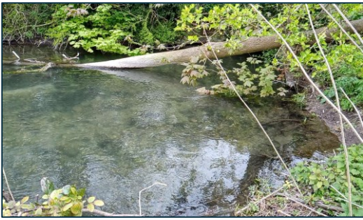
Fallen tree and back water downstream of culvert under Centurion Way.
