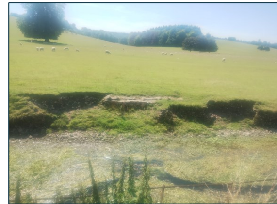
Left hand bank of river poached and partly reinforced.
